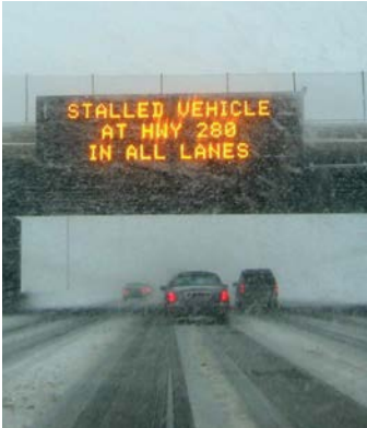
A dynamic message sign alerts drivers of an incident ahead.
